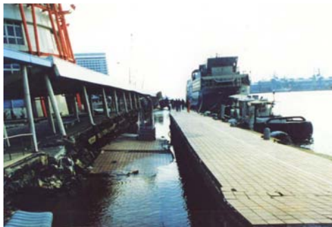
Photo.1 Damage of pile-type wharf
